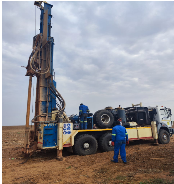
Figure 1. Start of drilling at the Bothaville Project in the Witwatersrand Gold Basin
